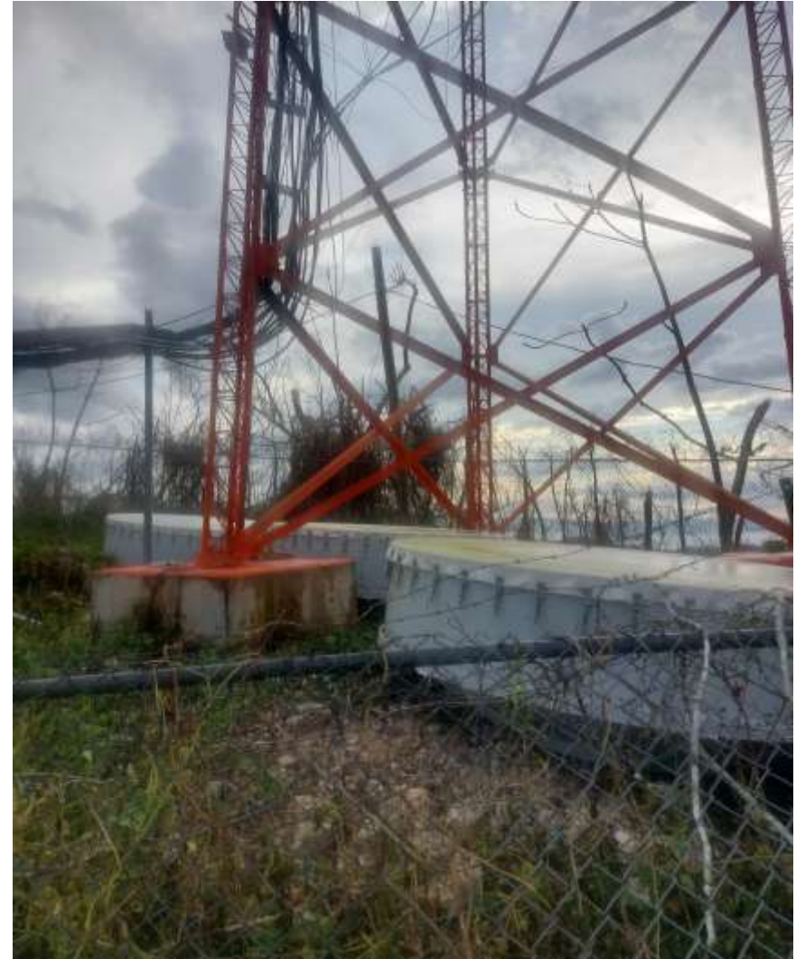
8ft Microwave Antennas down at the site
